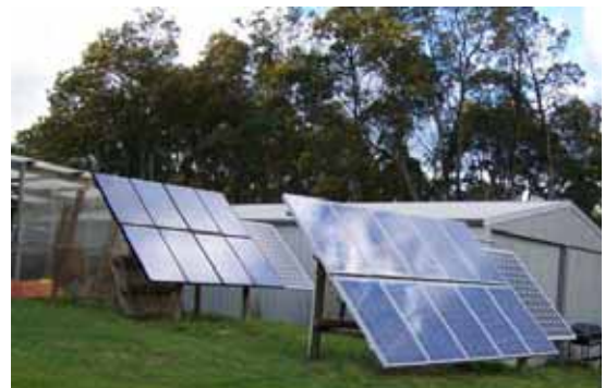
Array of John O'Grady's solar panels
